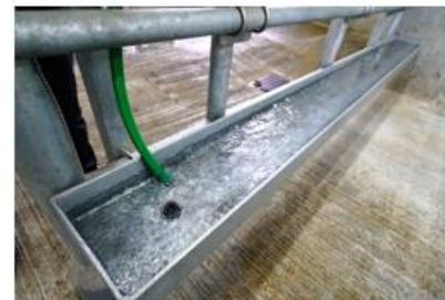
STARZEN MEAT PROCESSOR Co., Ltd. Akune Plant's drinking water system
