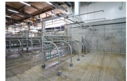
STARZEN MEAT PROCESSOR Co., Ltd. Akune Plant's berthing facility with misting system
